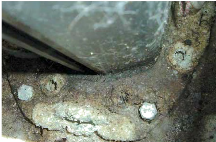
This mast footplate was not insulated from the mast or not bonded to the grounding system and was destroyed by stray current corrosion. Source: BoatUS.
